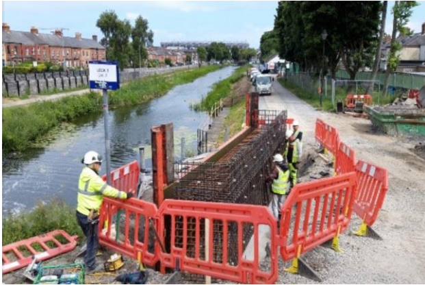
Image 3. Progress photos of the works being carried out as part of the Royal Canal Greenway Phase 3 as ramp beams were installed near Croke Park
