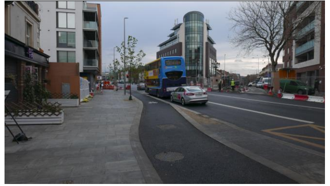
Image 2. Works progressing well on the inbound section of the Clontarf to City Cycleway at Five Lamps
