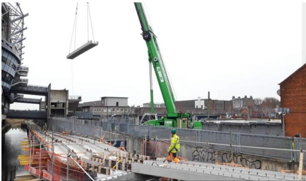
Image 4. Progress photos of ramp installation as part of the Royal Canal Greenway.
